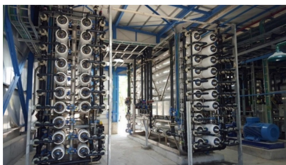
Fig. 1. Adama RO units (new trains)
