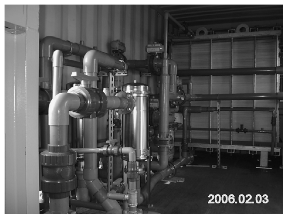
Fig. 4. Picture of EDR mini-plant installed in a container.
