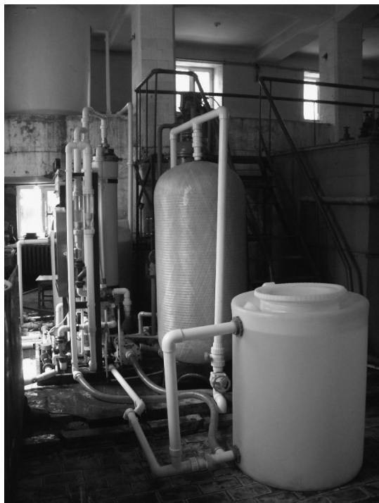
Fig. 2. Photo of the 120 m 3 /d pilot plant.
