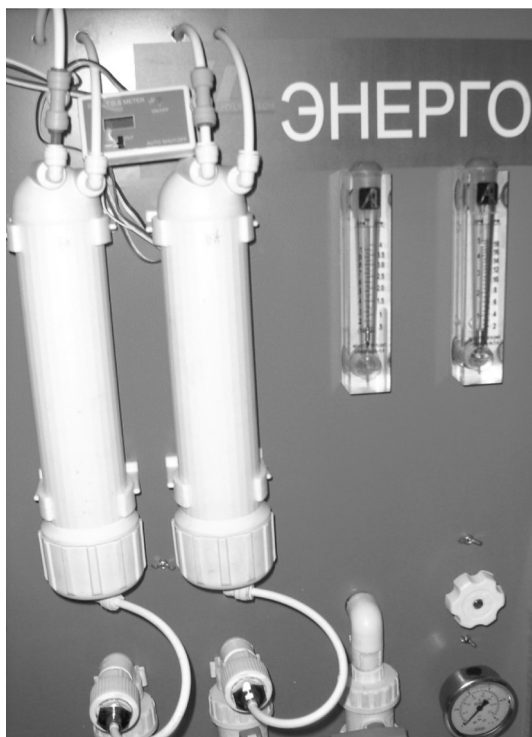
Fig. 2. Spiral-wound membrane modules of NF/RO unit.
