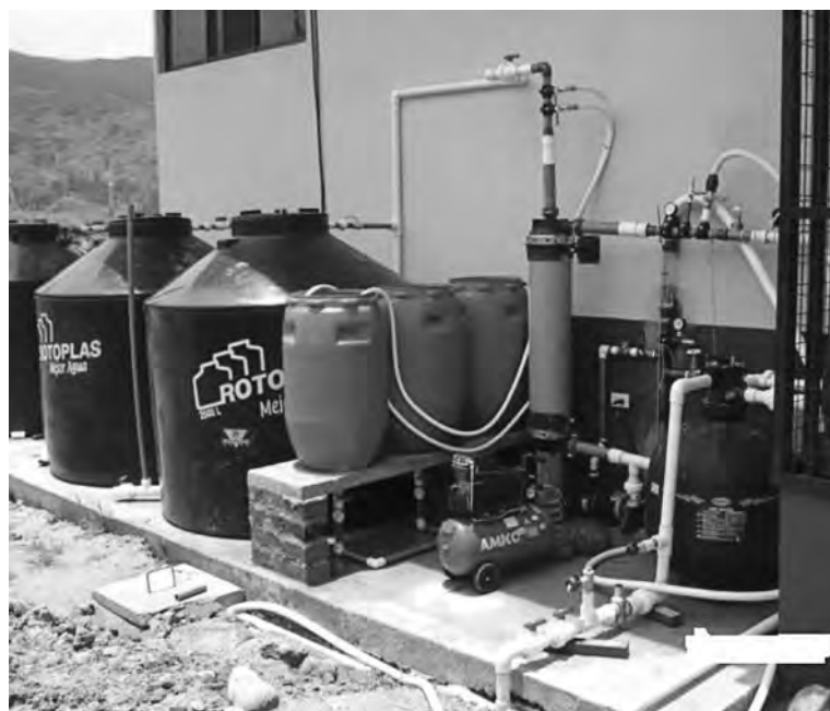
Fig. 2. Picture of the system installed in Giron.
