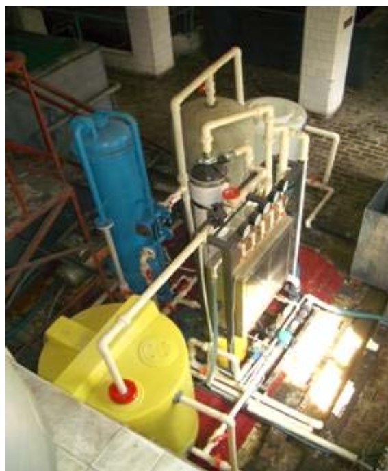
Fig. 2. Photo of the 120 m 3 /d pilot plant.
