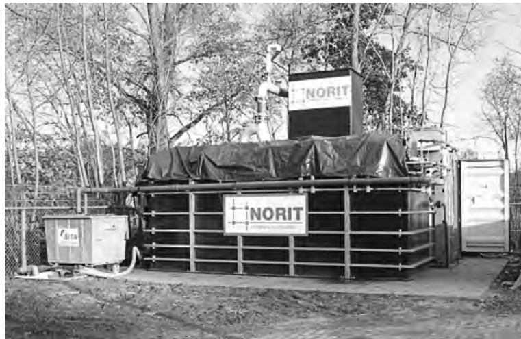
Fig. 5. AirLift MBT pilot at WWTP Ootmarsum.
