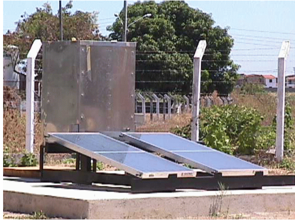
Fig. 1. Photo of the desalination system powered by solar collectors.
