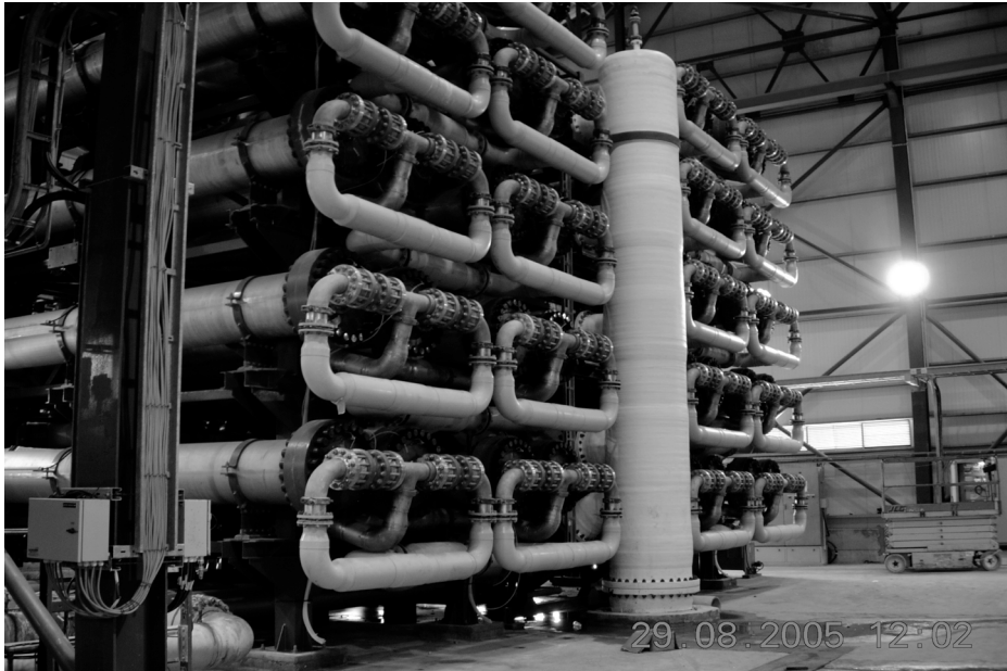
FIG. 11.14 Picture of DWEER pumping- power recovery device at the seawater RO Ashkelon plant (courtesy of Israel Desalination Engineering).
