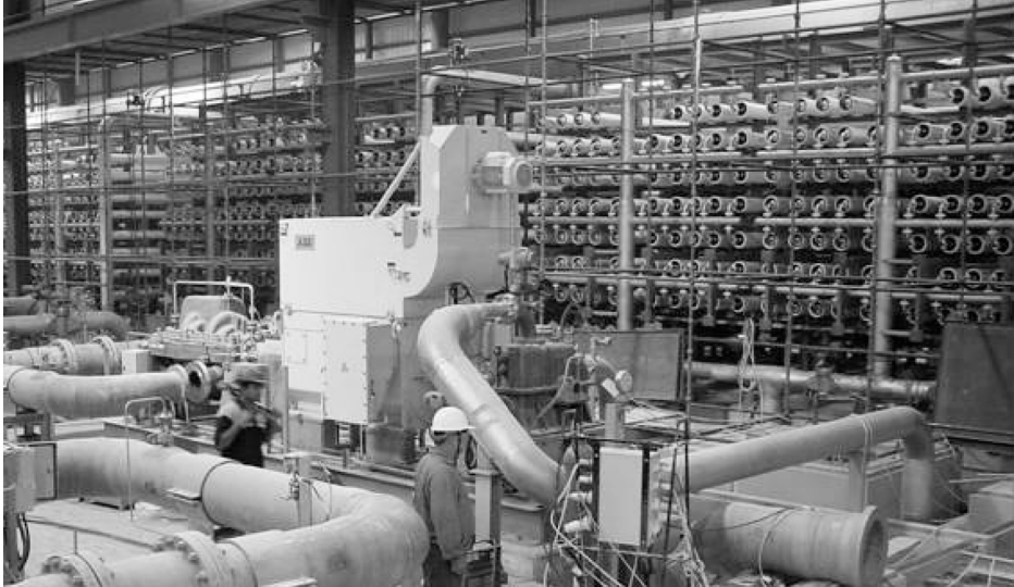
FIG. 20.24 Fujairah plant SWRO racks and feed pump/ER turbine arrangement.
