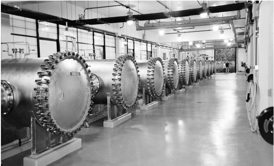
FIG. 8.3 Battery of cartridge filters housings in horizontal configuration.
