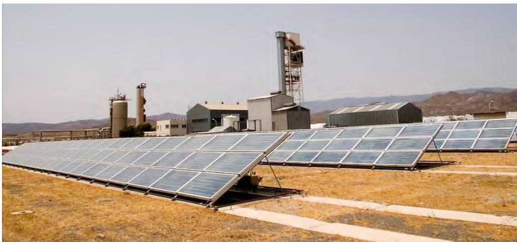
AQUASOL solar distillation plant at PSA
