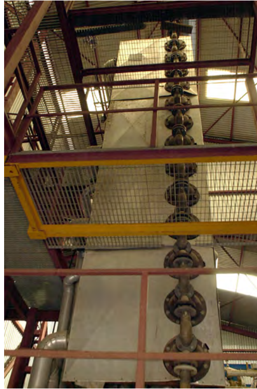
AQUASOL solar multi-effect distillation plant at PSA
